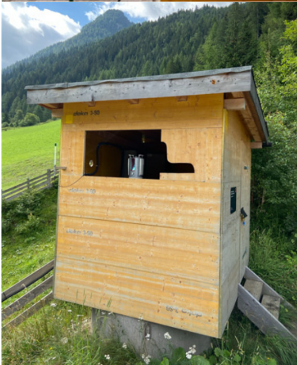
Figure A4. System installation in Vals. Pillar and shelter.
